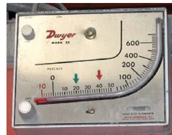
Booth manometer, useful for detecting blocked filters or poor ventilation flows.
