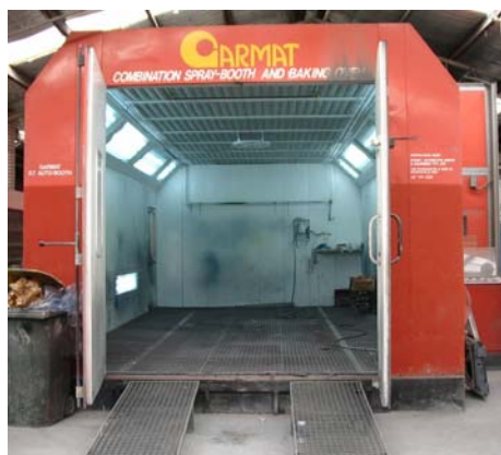
A properly designed and well-maintained spray booth ensures efficient capture of spray painting emissions
